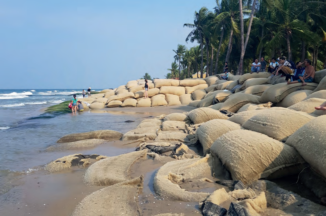
Fig. 138 | Current protection system against sand beach slides at Hoi An Beach. 2019. (own)
